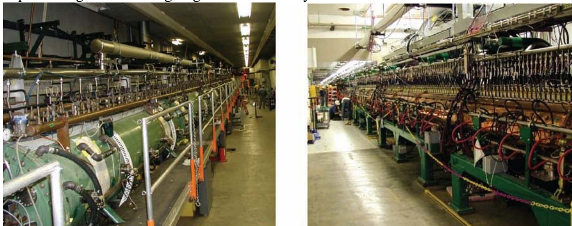
Fig. 4. Photograph of (a) the LANSCE-DTL water-cooling systems and (b) similar SNS-DTL systems.
