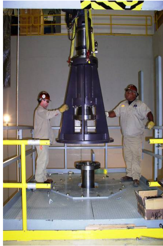
Figure 5. Installation of the rotating target drive module on the in-place target module.
