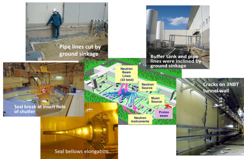
Figure 4 Damages around MLF: Subsidence with 1.5 m depth, inclination of liquid nitrogen tanks, cracks on the wall of 3NBT tunnel, broken shutter flanges, seal bellow elongation of target vessel, etc.
