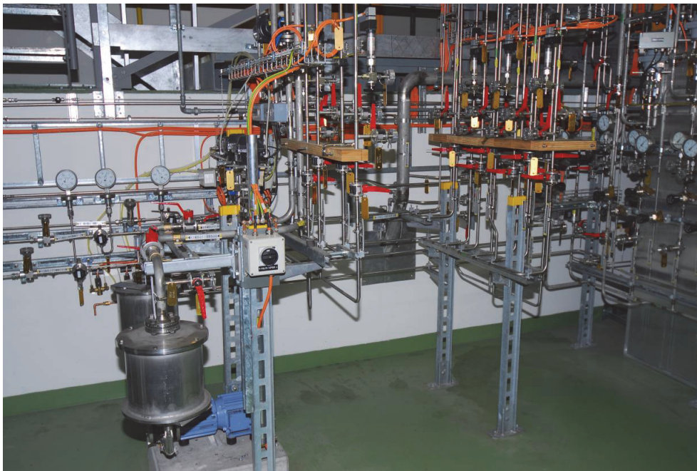
Figure 4. “Helium2” as an example of the installations in the gas central for maintaining and monitoring the controlled atmosphere for the neutron beam ports.
