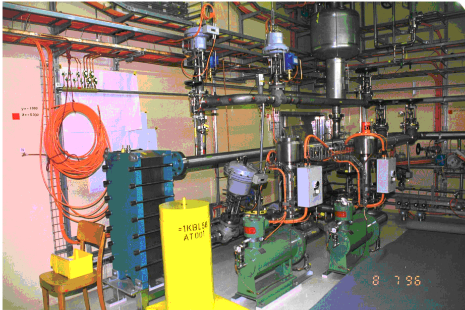
Figure 2: The installations of the target D2O cooling loop in the cooling plant room
