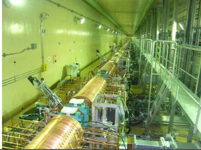
Figure 1. The linac accelerator tunnel after installation of ACS cavities.
