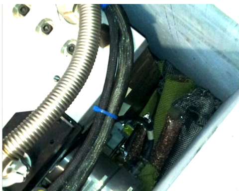
Figure 7. Bags with copper as an additional shielding at CNCS
